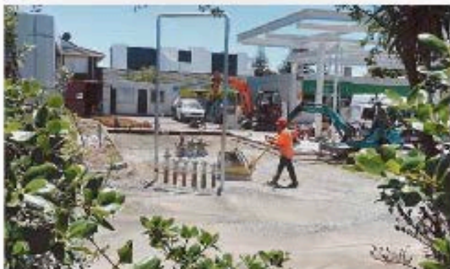
The structure in the foreground, at BP Orewa, will support six fuel vent pipes, potentially sending petrol fumes in the direction of neighbouring houses.
